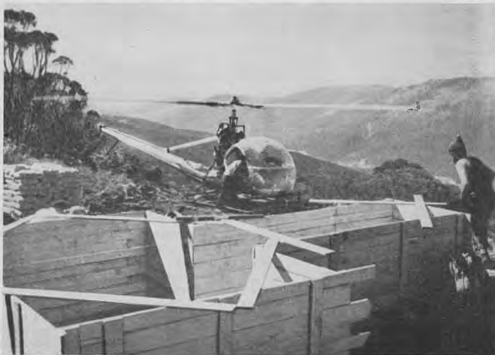
Helicopter transport of cement to the top station of Thredbo Chairlift, Easter, 1958.
