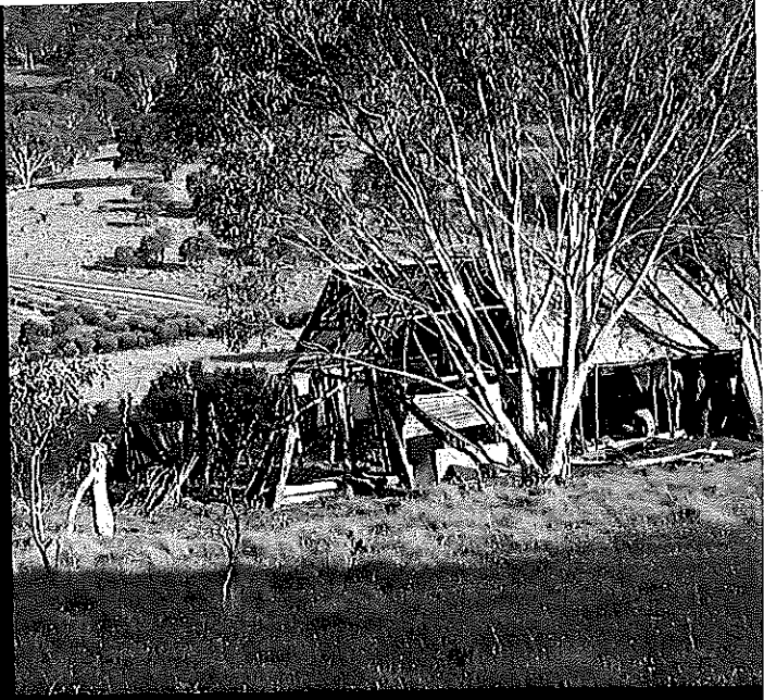
Spencers Hut: not on the demolition list, but on its last legs and will probably soon be gone anyway. Near Coolamine Caves.
